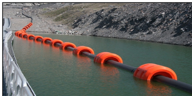
Hanging / Floating - Pipe Line
