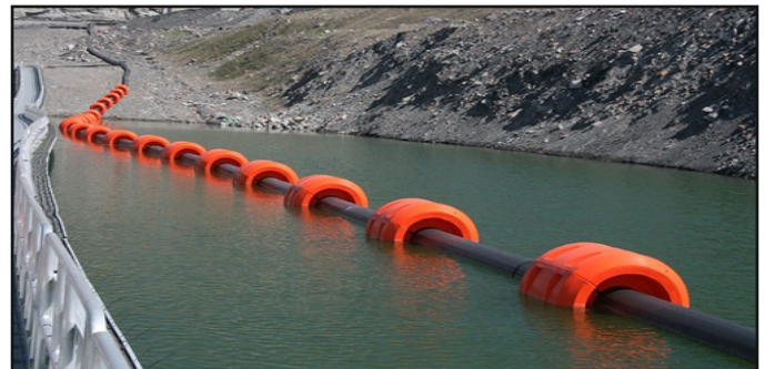
Hanging / Floating - Pipe Line
